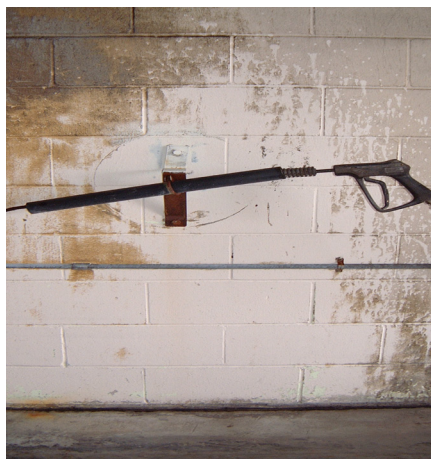
Block wall — applied TCI 303 H.D. as a demo to bottom of wall
