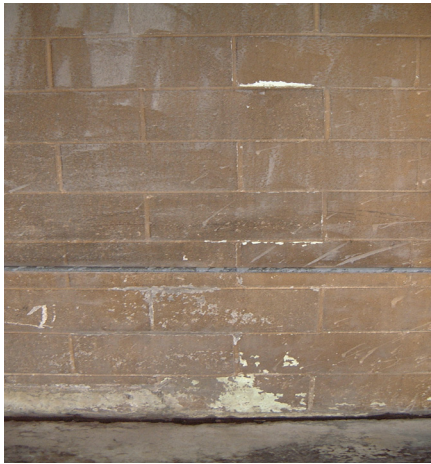
Block wall — accumulated scum
