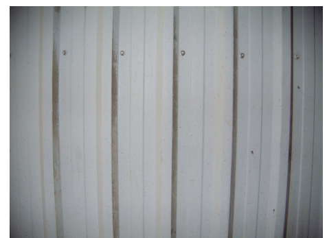
Garage Wall - Exhaust Soot - After
