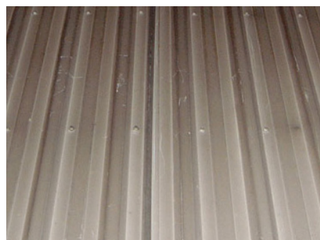
Garage Wall - Exhaust Soot - Before
